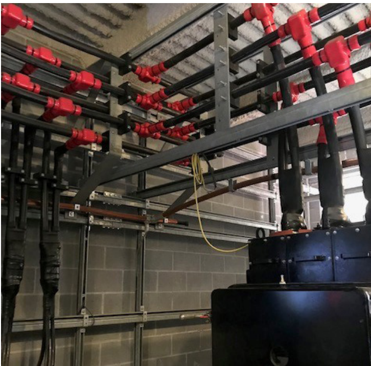
Figure 1: 480V secondary cables and transformer (Courtesy of www.impactaconsulting.com )
