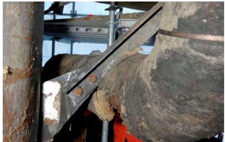
Figure 2: The proximity of the corroded pipe to the walkway bracket
