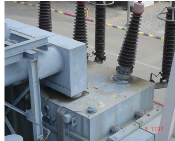
Figure 4: Step-up transformer nitrogen blanket leak
