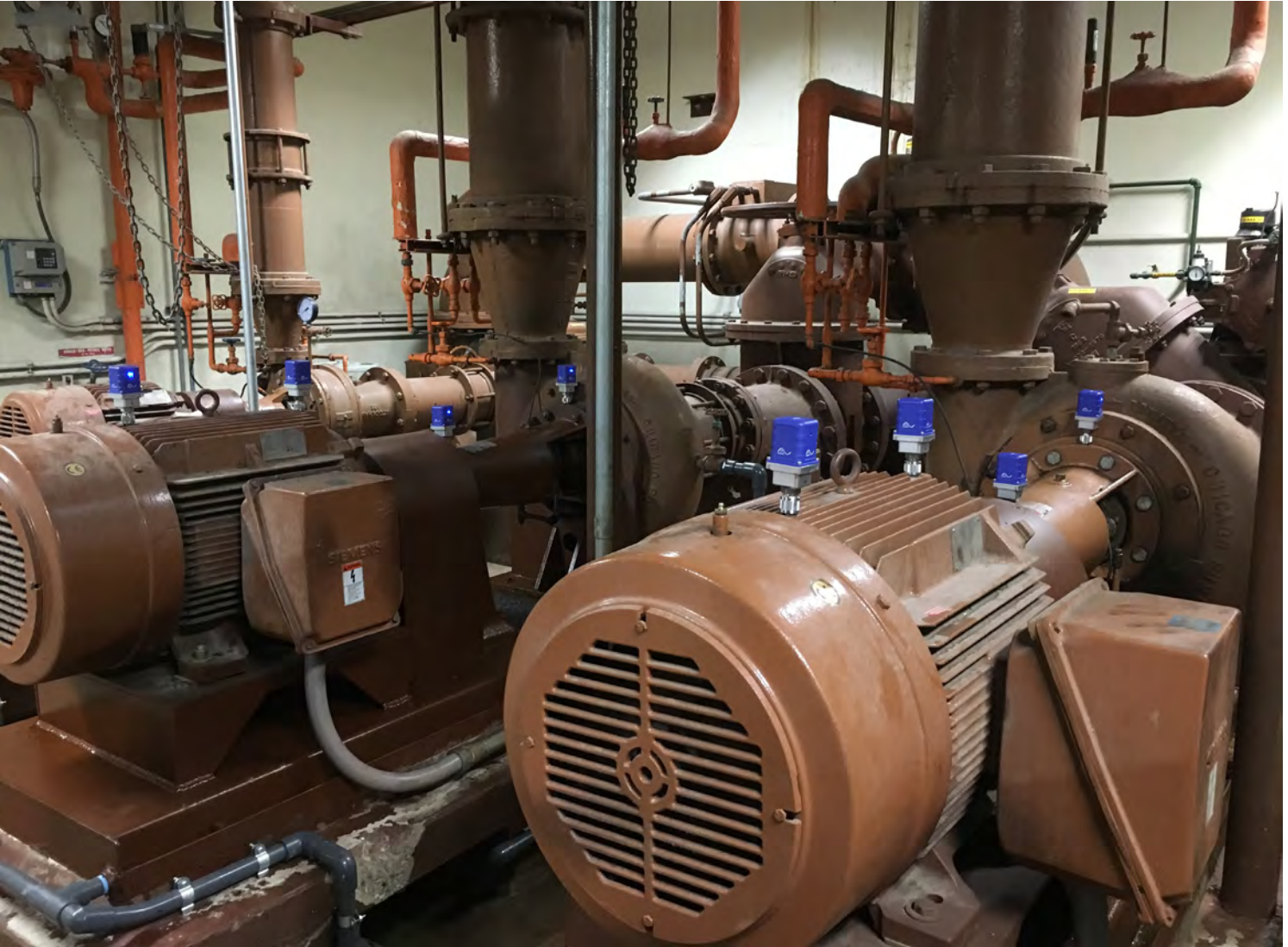
Figure 3: Mechanical diagnostics enabling PdM at a wastewater facility
