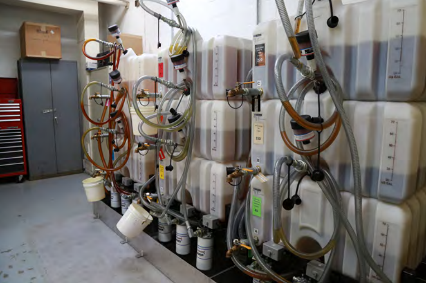
Figure 3: DC Water's lubricant storage
