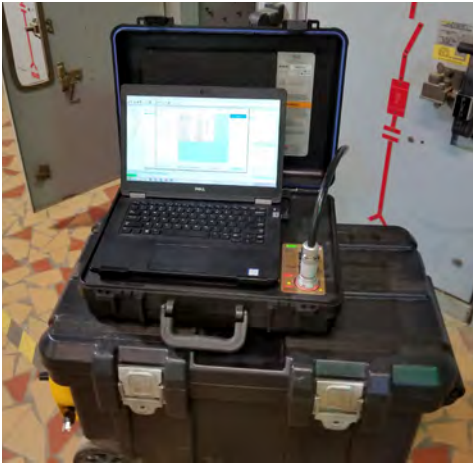
Figure 1: De-energized testing is important as it provides an opportunity to test insulation
